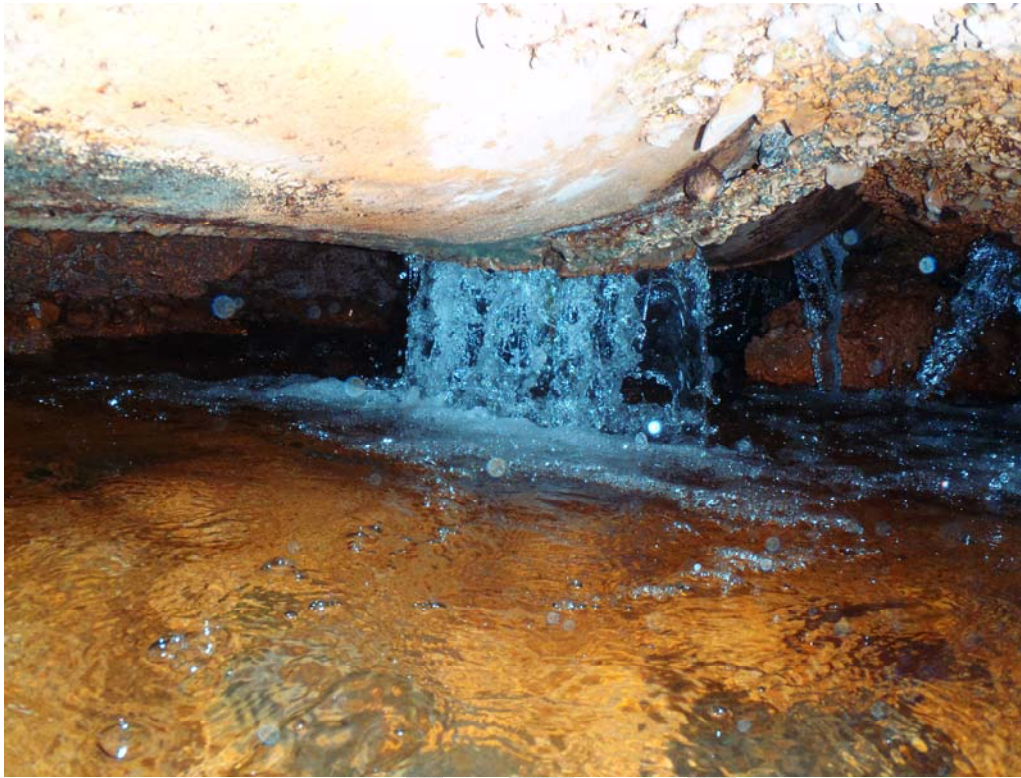
Figure 4. Damage to new culvert from June 2010 flood (photo courtesy of Nathan Pence).
