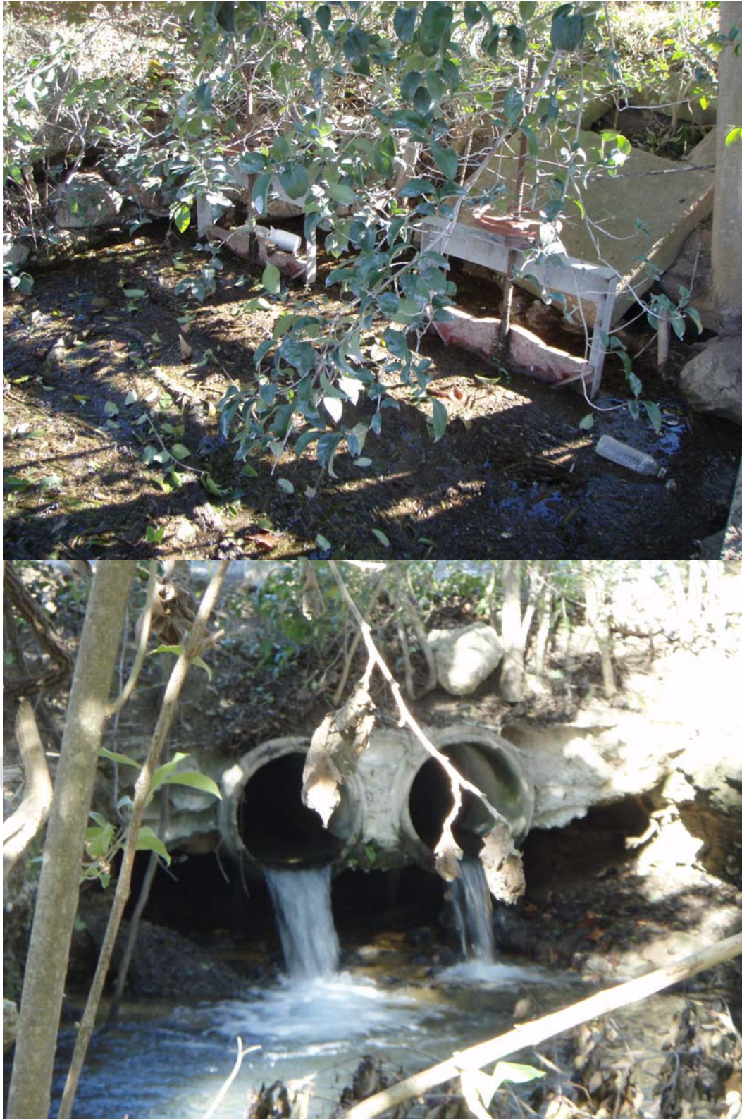
Figure 3. Old set of 24-inch culverts with limited capacity in the Old Channel.
