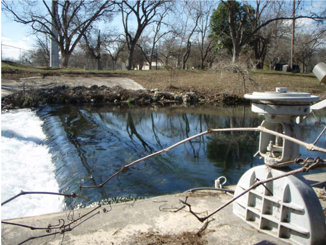
Figure 5. Reconstructed LCRA weir across from Landa Park office.
