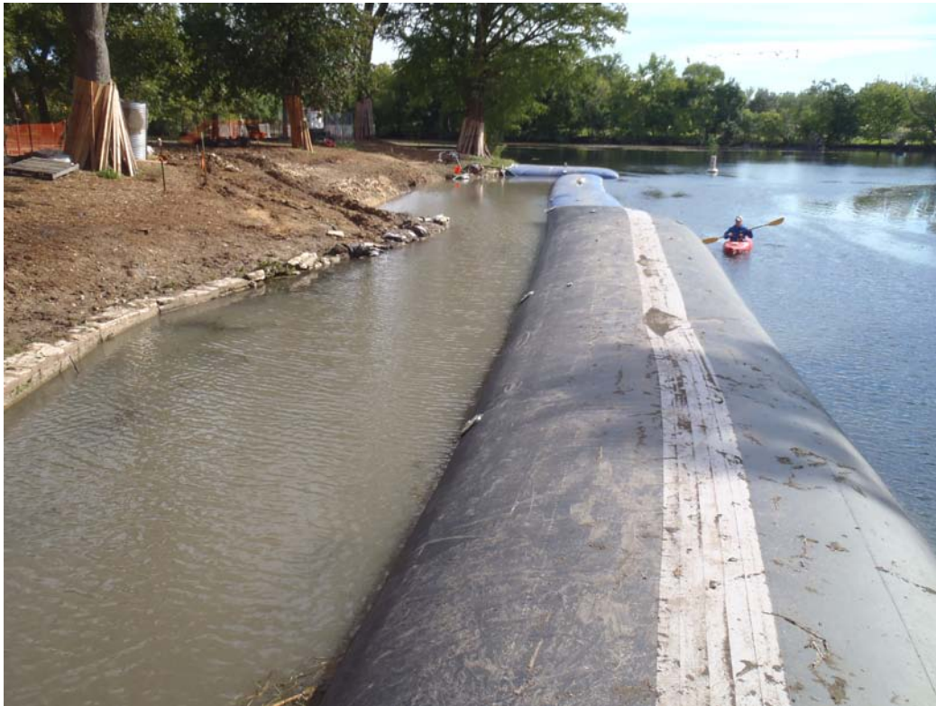
Figure 5: Landa Lake walls construction project - downstream view towards the lake. Note larger black inflatable coffer dam.
