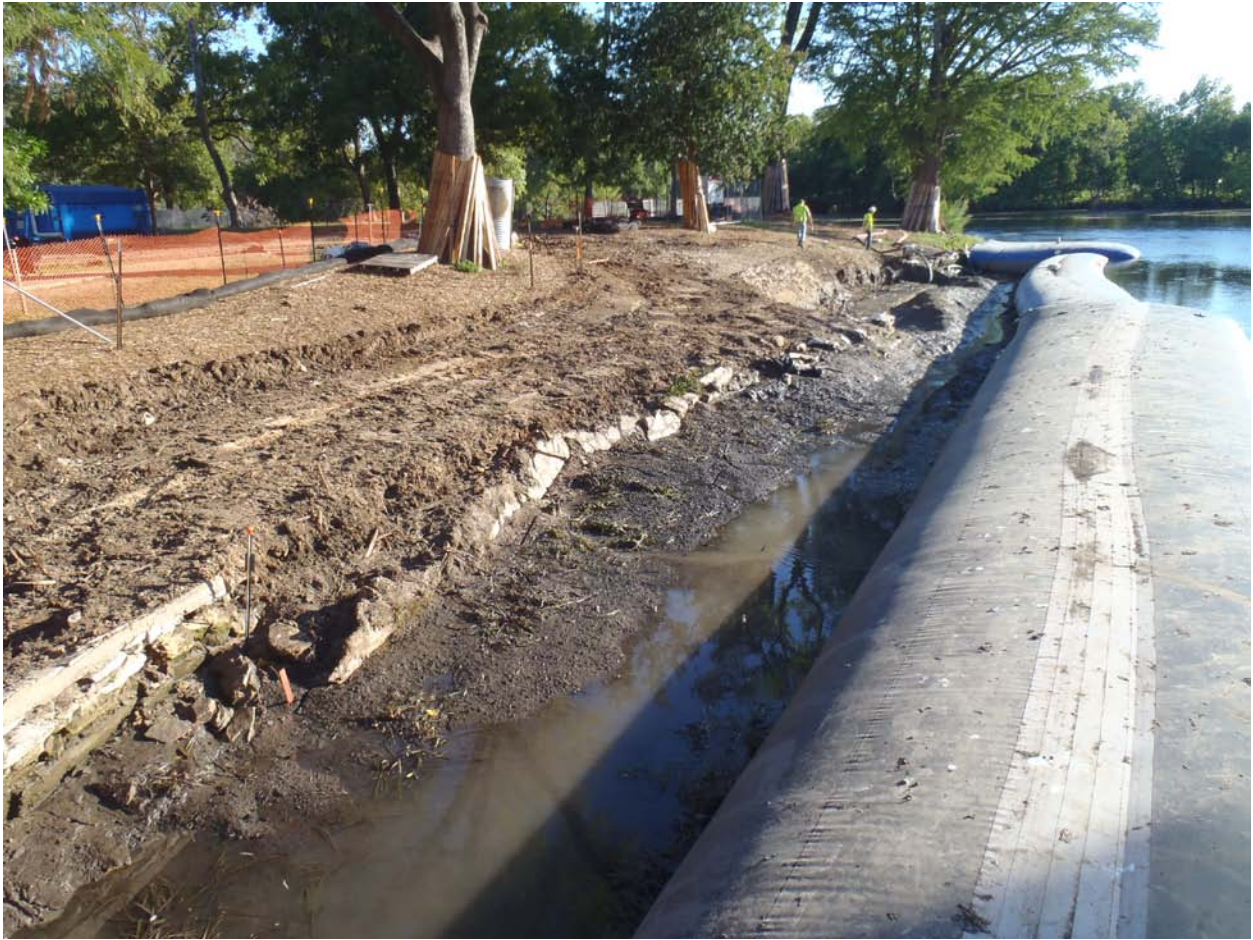
Figure 5: Landa Lake walls construction project - downstream view towards the lake. Note top of photo shows the old walls removed with the lower part of the photo showing the old walls needing to be removed.
