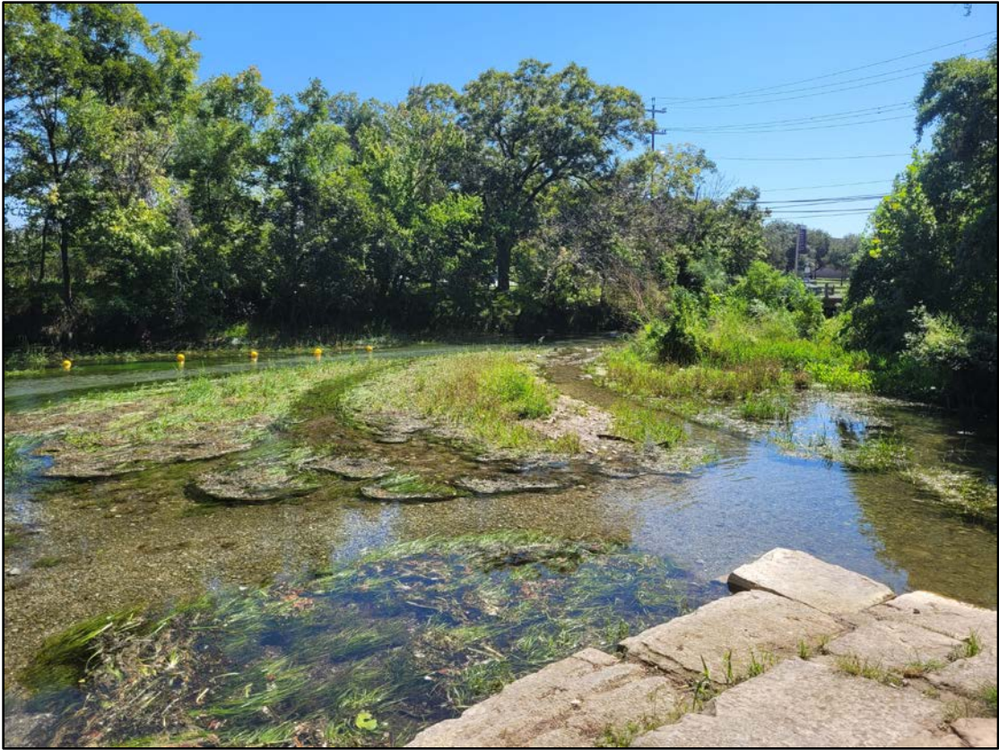
Figure 6: Spring Lake Dam Sessom's Island on September 28, 2022.
