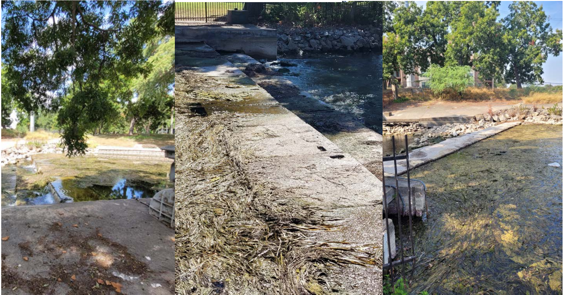
Figure 13: New Channel Park Office Weir on July 25, 2023 (~85 cfs – left [flow over weir], August 10 (~70 cfs – center [trickle of water flowing over weir] and August 21 (~60 cfs – right [no water flowing over weir – only seepage through dam]).
