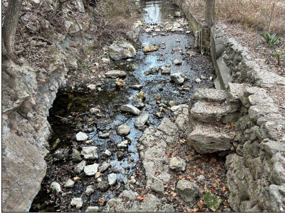
Figure 7. Reduced flow at Spring Run 3 at ~70 cfs on February 10 th , 2026.
