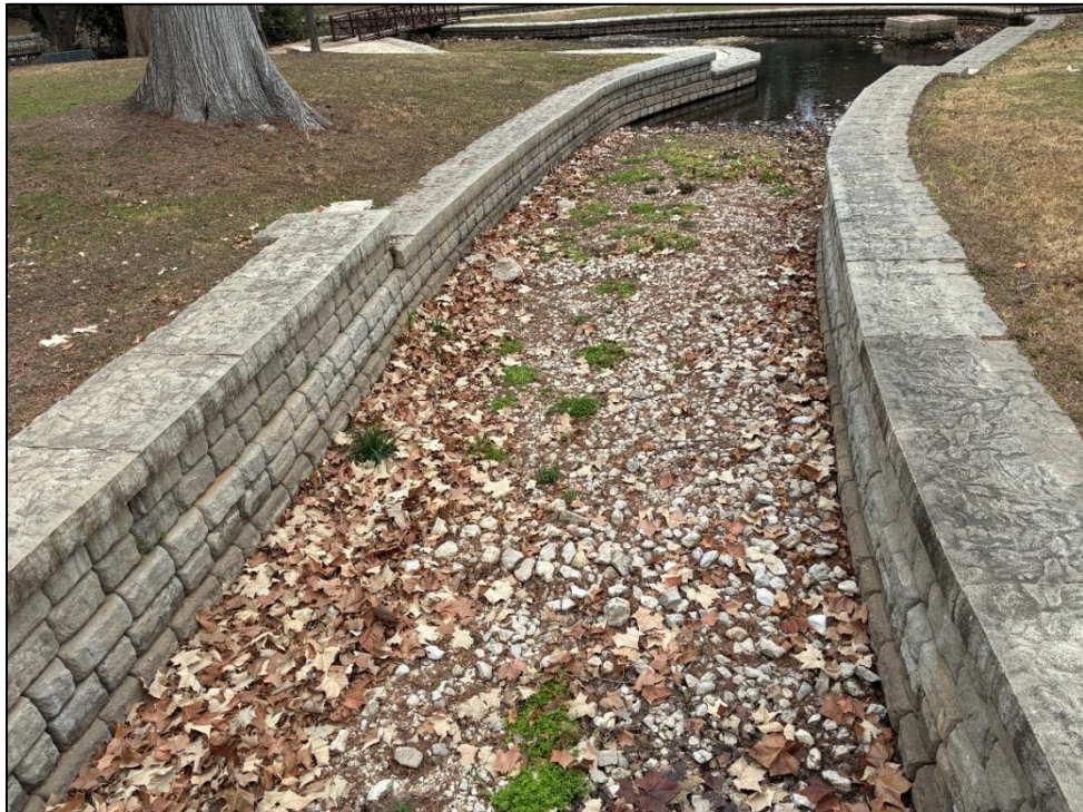
Figure 6. Dry area at Spring Run 2 at \sim 70 cfs on February 10 th , 2026.
